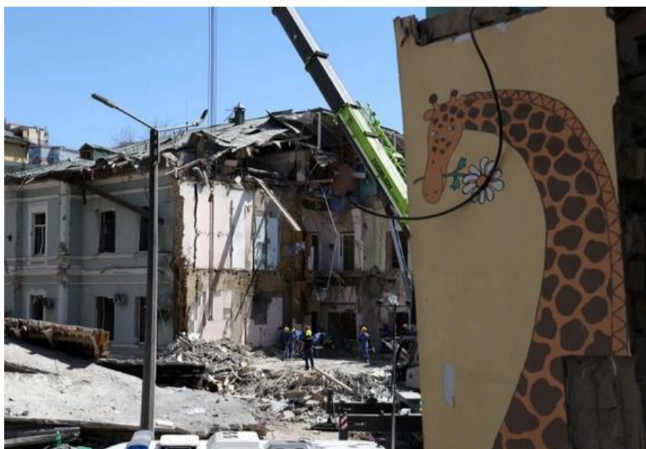
Rescue personnel operate and clear the rubble of the destroyed building of Ohmatdyt Children's Hospital, a day after a missile attack in Kyiv during the Russian invasion in Ukraine. Targeting hospitals in Ukraine is a "war crime," a senior UN official told an emergency meeting of the Security Council on Tuesday in the wake of deadly strikes that Kyiv blamed on Russia. (Photo by Anatolii STEPANOV / AFP)
